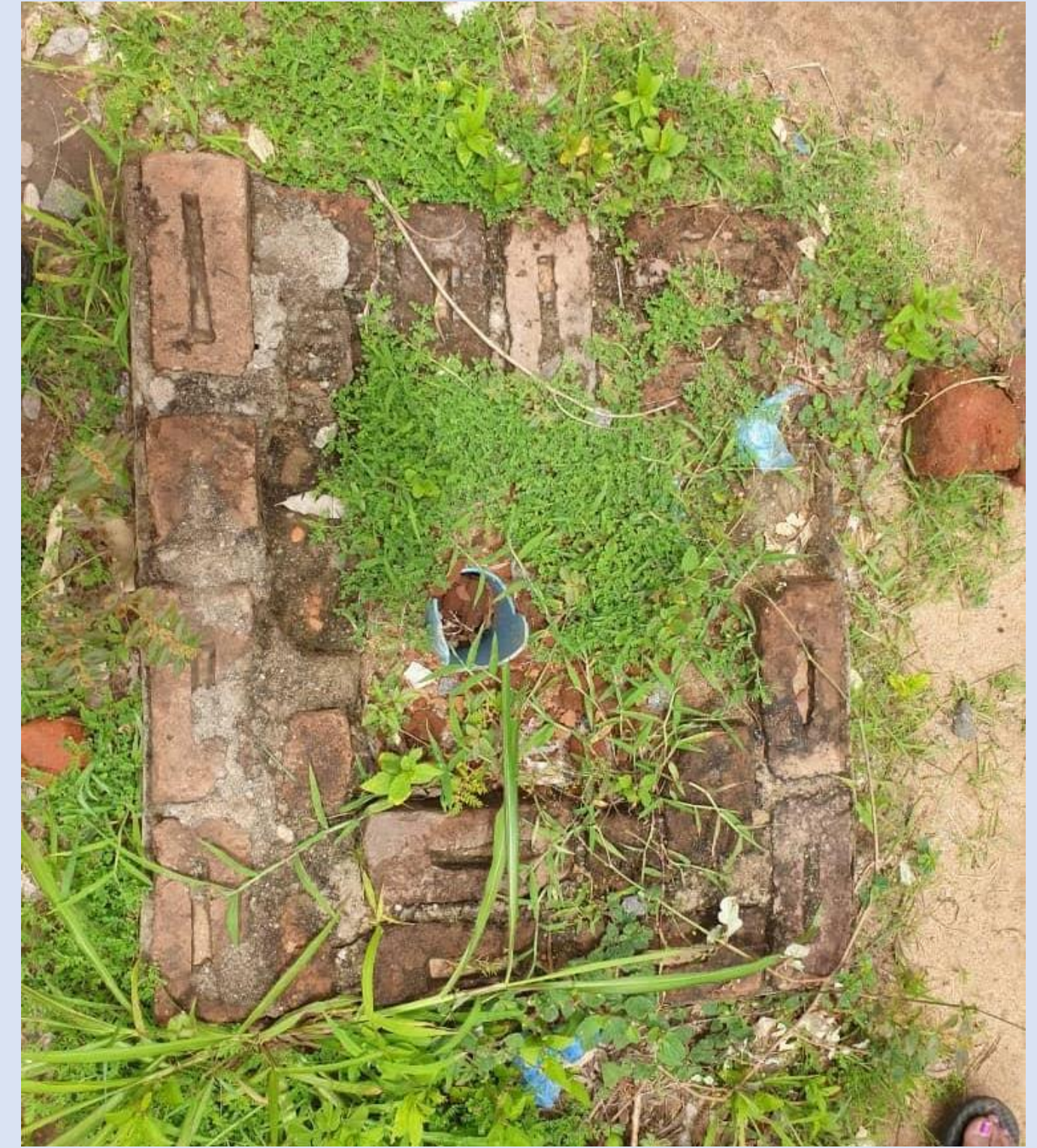
Figure 2. Image of a non-functional groundwater monitoring point. The monitoring point has been vandalised by local community. (Government of Malawi et. al, 2022)
